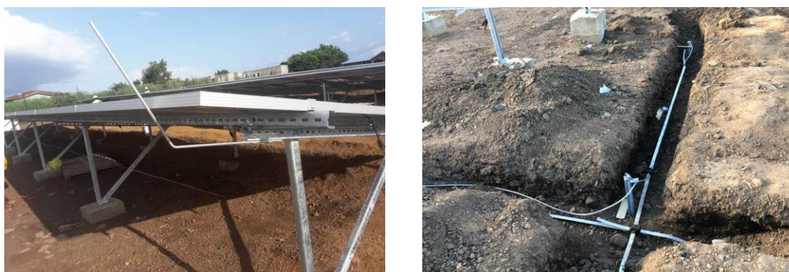
Figure 3: Solar panel mounting system showing lightning protection above and below ground
